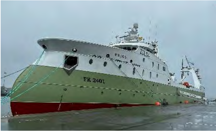
The JSMEA delegation observes a fishing trawler vessel under construction at Astilleros Nodosa.
